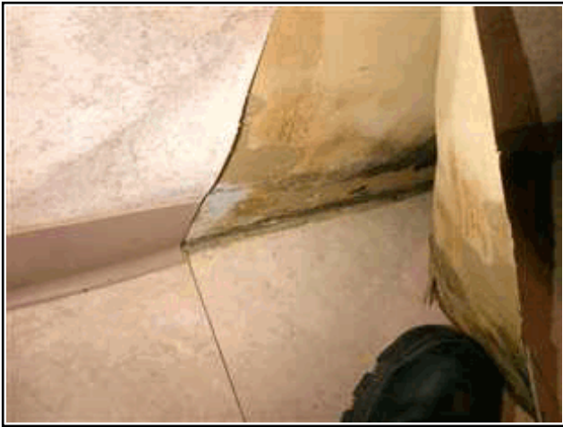
Room 286 - Bathroom mold.jpg
