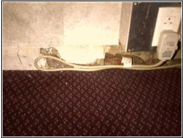
Room 277 - Hole in wall near heating unit.jpg
