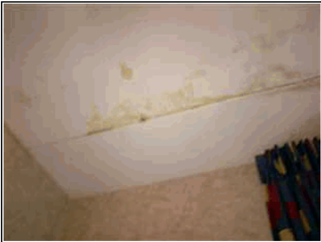
Room 277 - Stained ceiling.jpg
