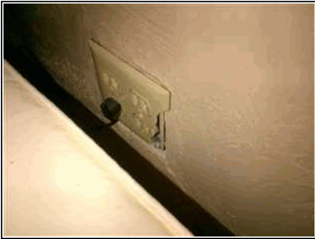
Room 170 - Broken outlet cover.jpg
