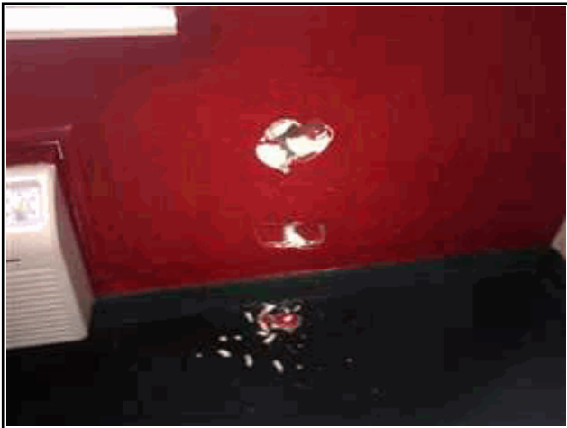
Room 285 - Holes in wall.jpg
