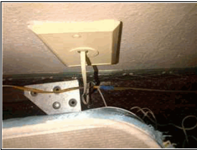
Room 180 - Spliced lamp cord.jpg
