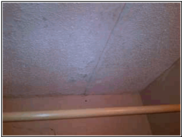
Room 159 - Mold on bathroom ceiling.jpg
