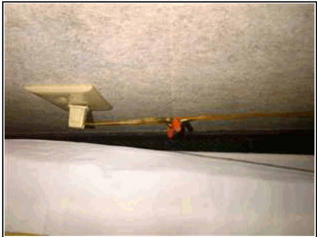
Room 287 - Spliced lamp cord.jpg
