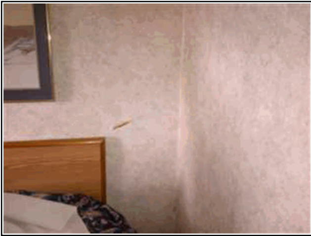
Room 288 - Stained Walls.jpg
