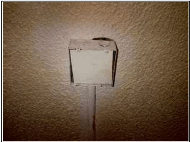
Room 187 - Unapproved cover plate.jpg
