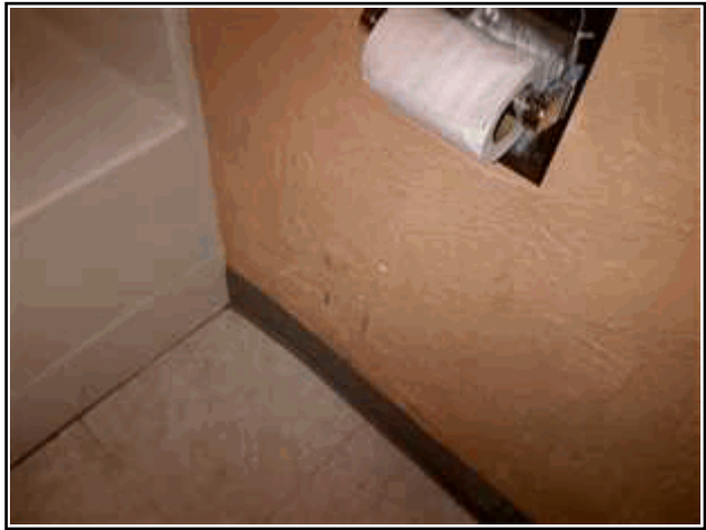
Room 164 - Stained bathroom wall.jpg
