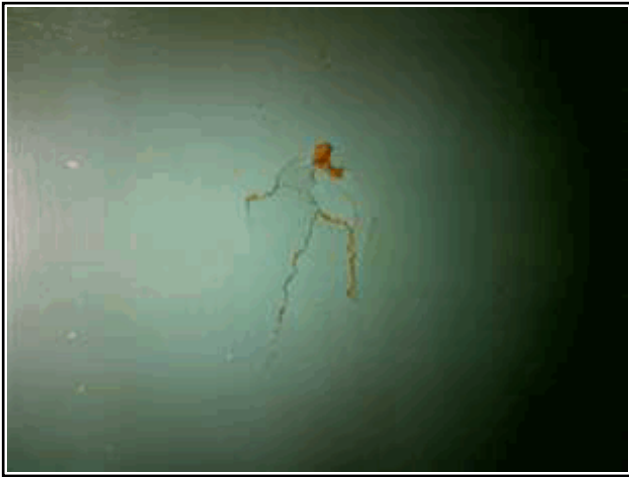
Room 278 - Hole in bathroom door.jpg
