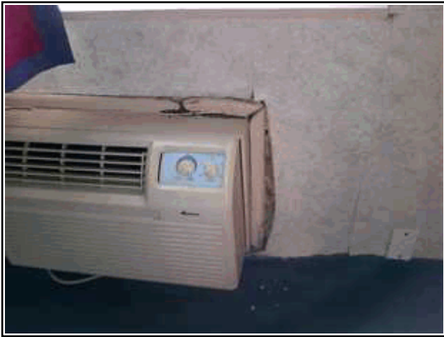
Room 272 - Rotting wood around heating unit.jpg
