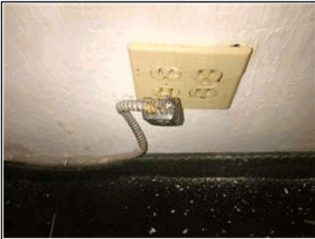
Room 182 - Broken outlet cover and exposed wires.jpg
