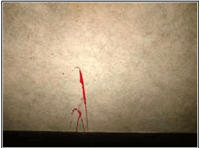
Room 275 - Stained wall.jpg
