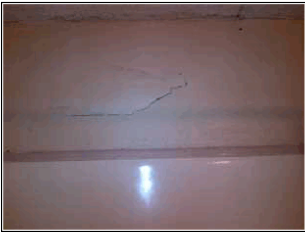
Room 159 - Damaged wall in bathroom.jpg
