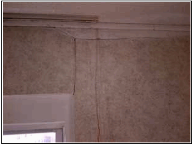
Room 286 - Stained Walls.jpg
