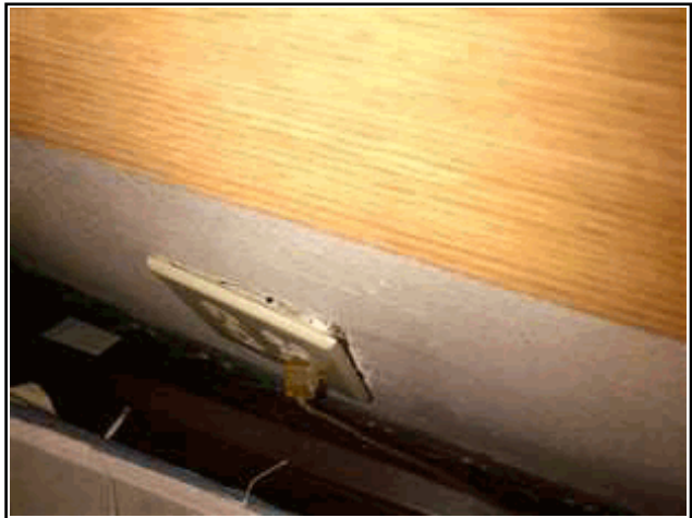
Room 180 - Outlet protruding from wall.jpg
