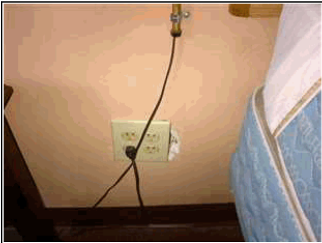
Room 279 - Hole in wall next to outlet.jpg
