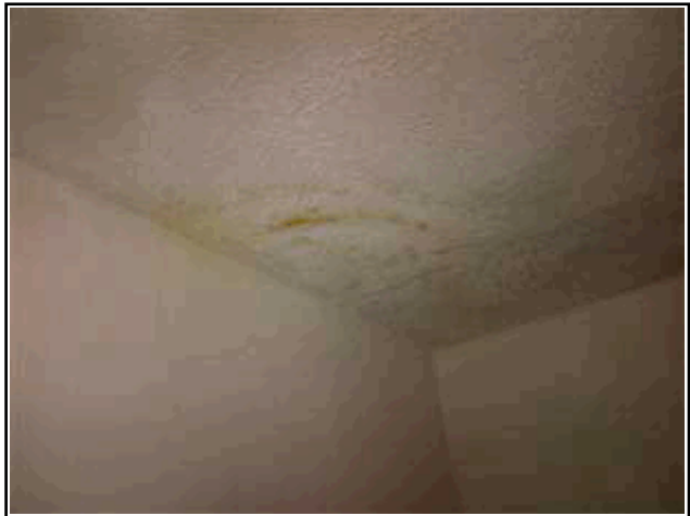
Room 283 - Stained Ceiling.jpg
