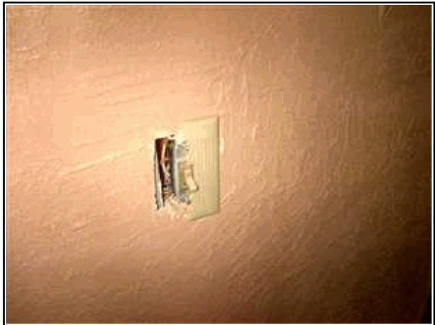
Room 164 - Broken light switch cover.jpg
