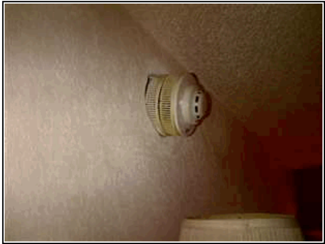
Room 187 - Hanging smoke detector.jpg
