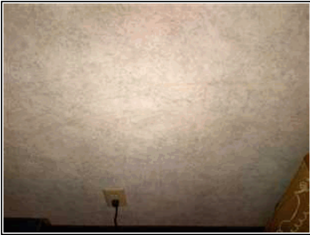
Room 278 - Stained wall.jpg
